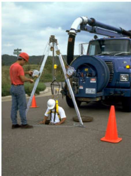
Figure 12-14 Effective vault rescue
