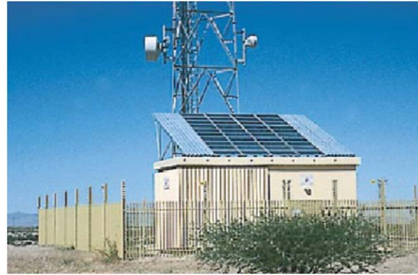
FIGURE 6 A telecommunication repeater station powered by a PV hybrid system.
