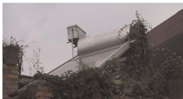
FIGURE 8 Flat-panel solar water heater, Yunnan province.
